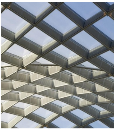
Figure 4.1 Detail of the Smithsonian Courtyard Enclosure designed by FP with SMG as consultant (source: http://www.fosterandpartners.com ).
